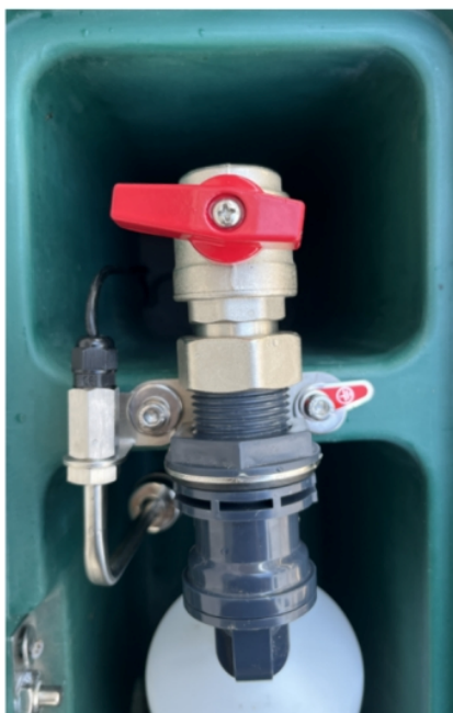
Shut-off valve SHUT
