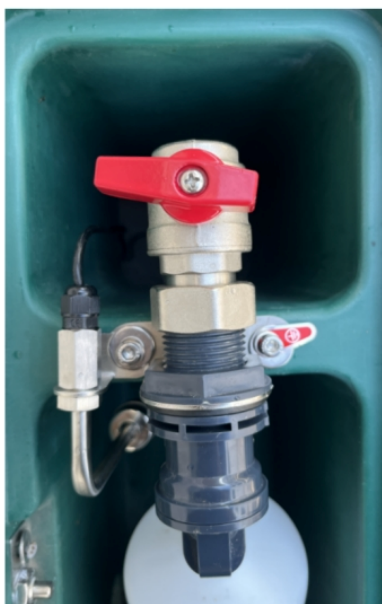
Shut-off valve SHUT
